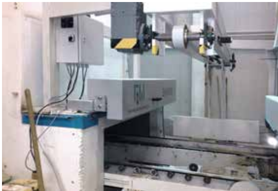
Height Control System and dumping station
